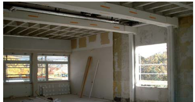
The much enlarged room on completion of works, with a far greater useable area exactly as the client required
