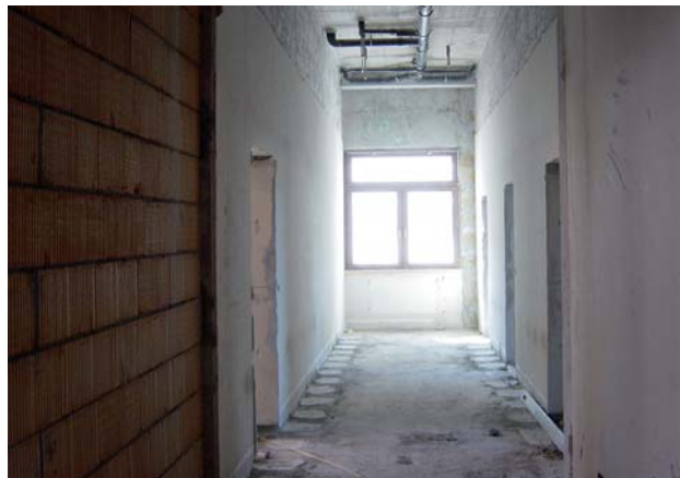
The two walls left and right of the window had to be removed
